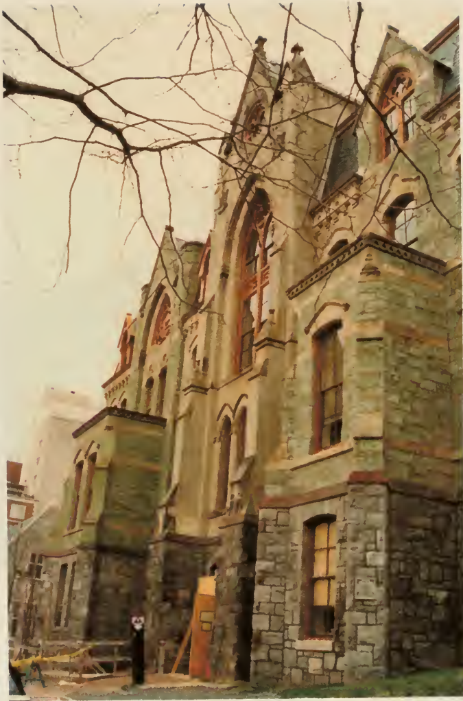
Photograph #37: East elevation of the East Wing of College Hall (1871-1872), University of Pennsylvania, Philadelphia. In urban settings, serpentine deteriorates badly. The University, in its desire to preserve the first building erected on its "new" campus in West Philadelphia, has undertaken to resurface the stone in an attempt to halt its deterioration. Unresurfaced serpentine stone can be seen in the middle of the photograph and the resurfaced stone can be seen on either side
